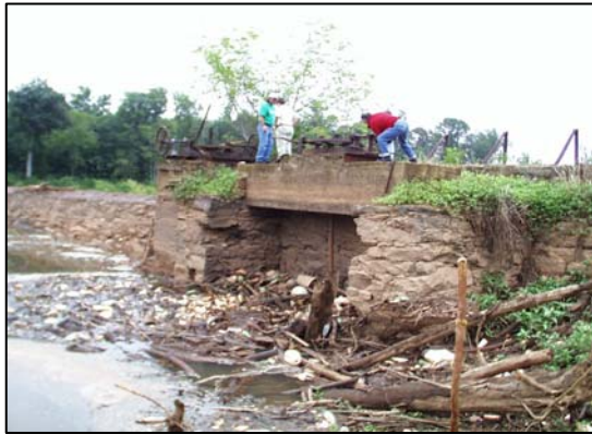
Photo 1: Lake Conestee Dam, ca. 1892, on the Reedy River, Greenville County. View of dam from upstream with partially open gate, August 2000. Note dilapidated gate assembly and accumulated trash and debris.
