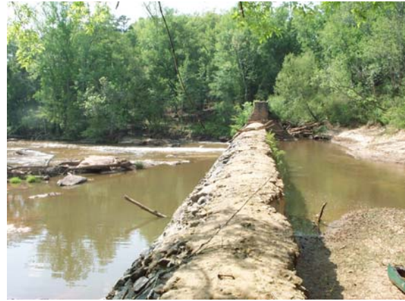
Photo 3: Cedar Falls Dam – note canoe in bottom right for scale. Lower Greenville County.
